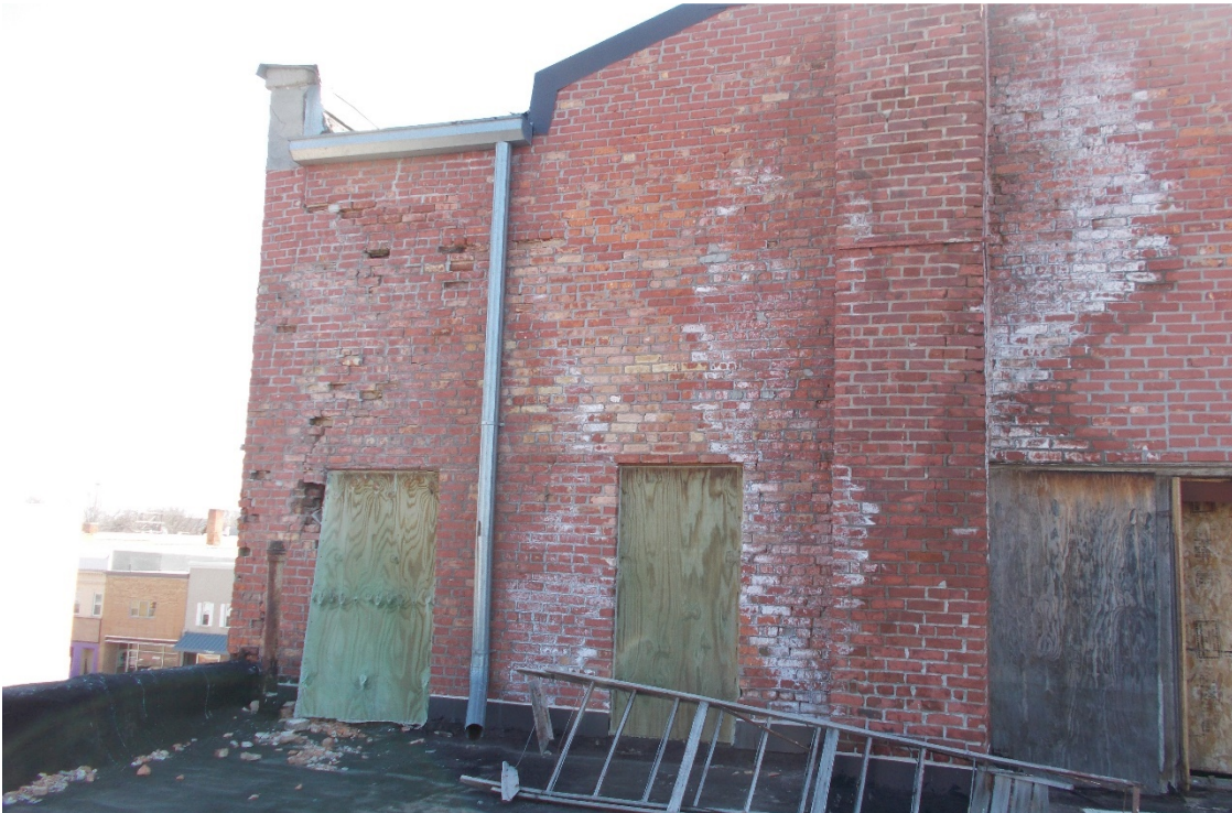
Figure 3. Photo showing deteriorated masonry along West wall of East building.
