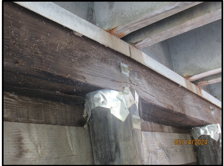
Crushing and Check Cracking North Abutment Cap over Pile 4
