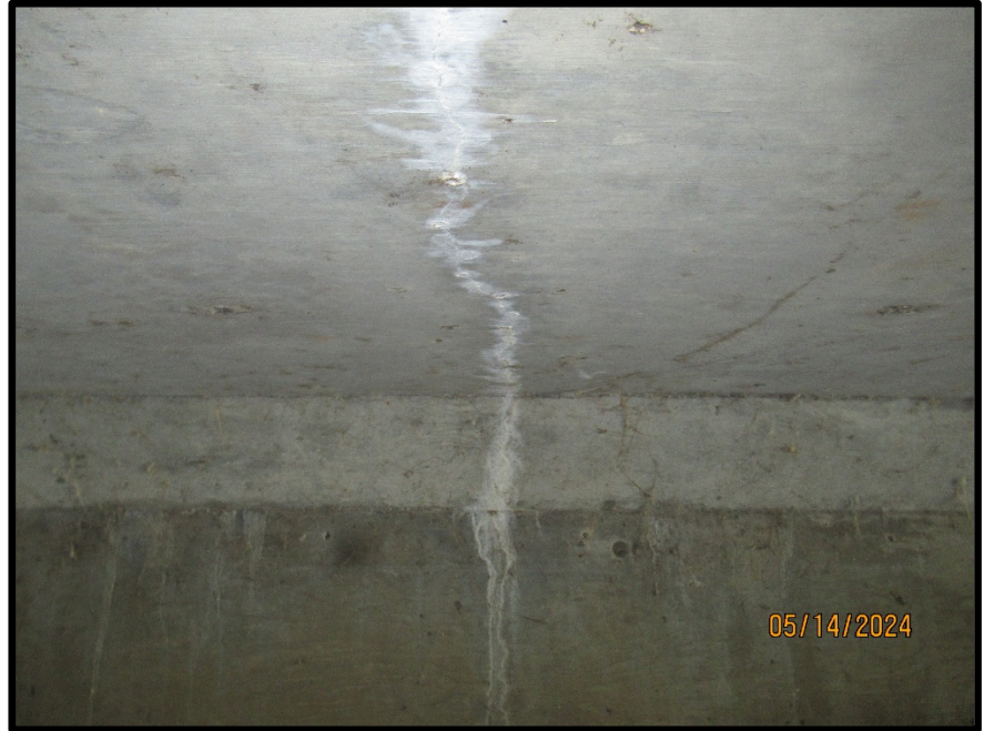
Typical Transverse Crack with Efflorescence in Top Slab of Barrels. East End of Barrel 1 Shown
