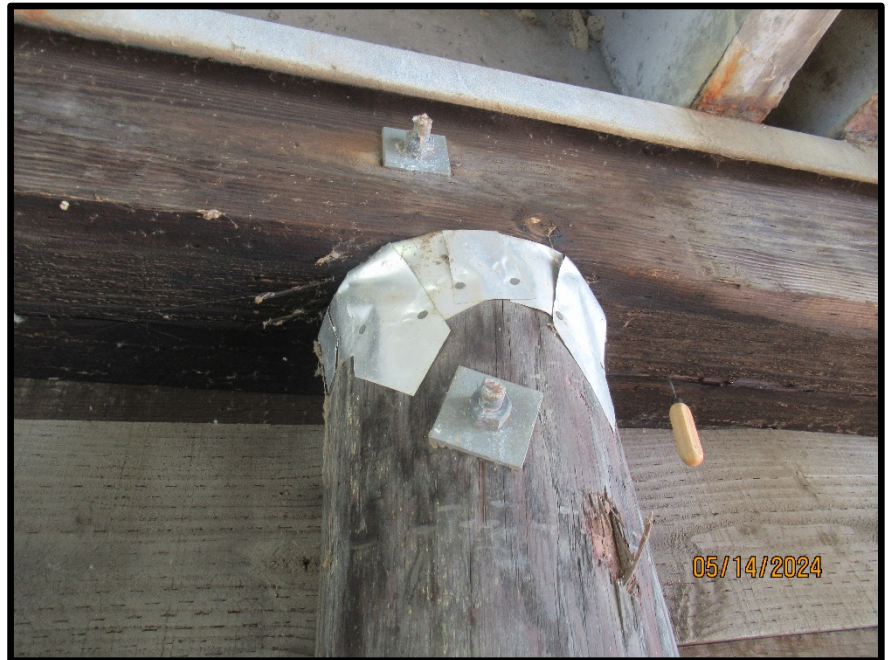
Crushing and Check Cracking North Abutment Cap over Pile 5
