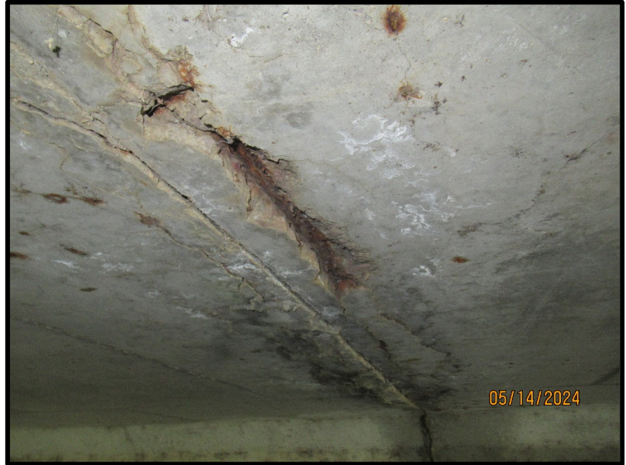
Cracking and Spall with Exposed Rebar in Top Slab of Barrel 1 at Construction Joint
