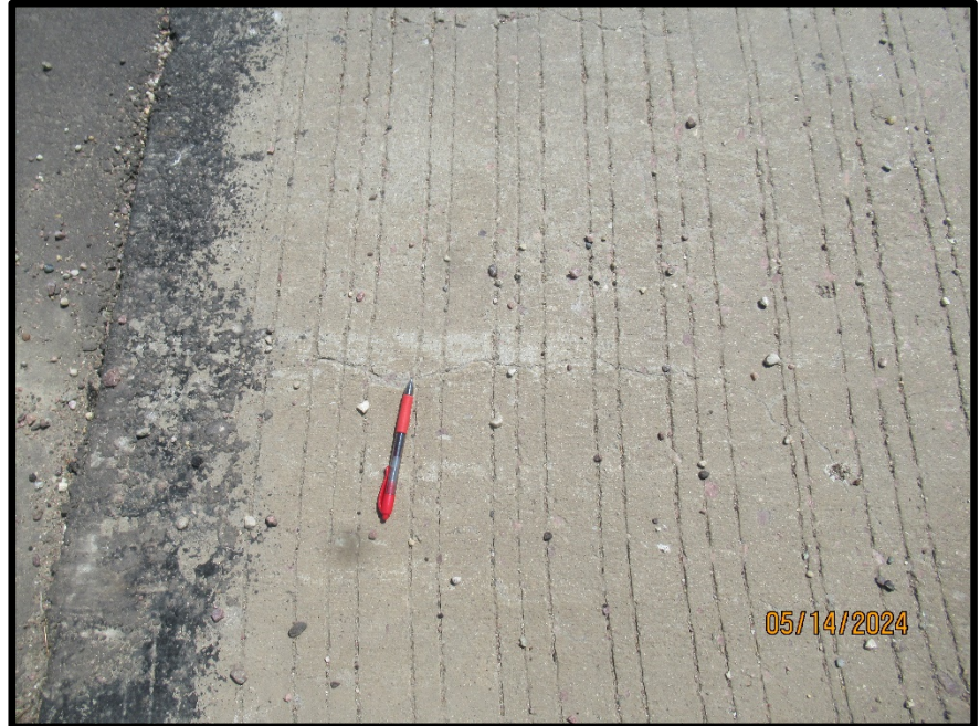
Light Longitudinal Cracking at North End of Bridge Deck
