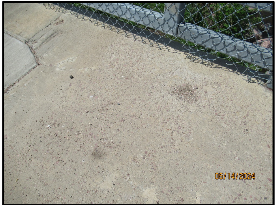
Scale and Cracking of Bridge Sidewalk at SW Corner
