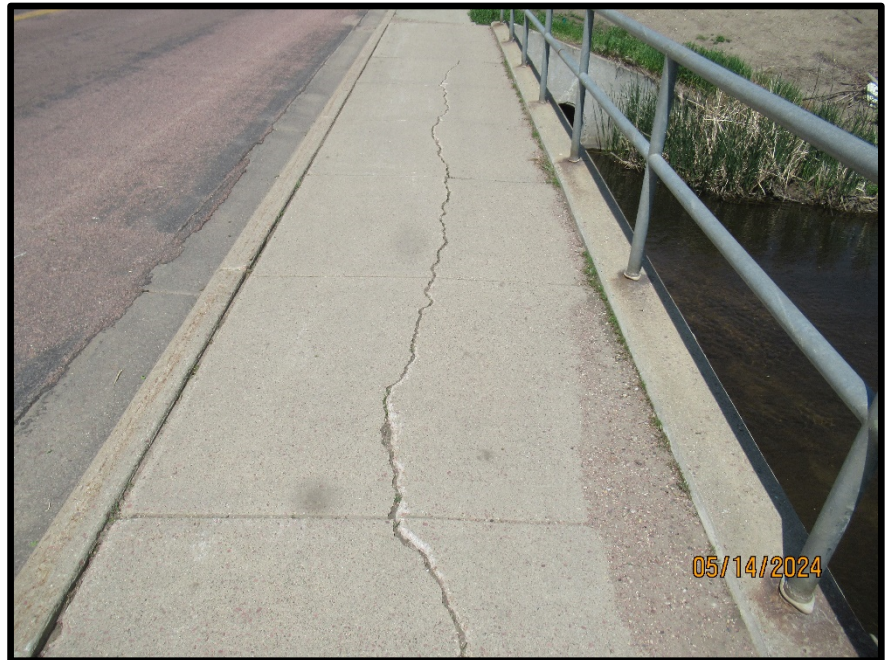
Longitudinal Crack in East Sidewalk with Humping
