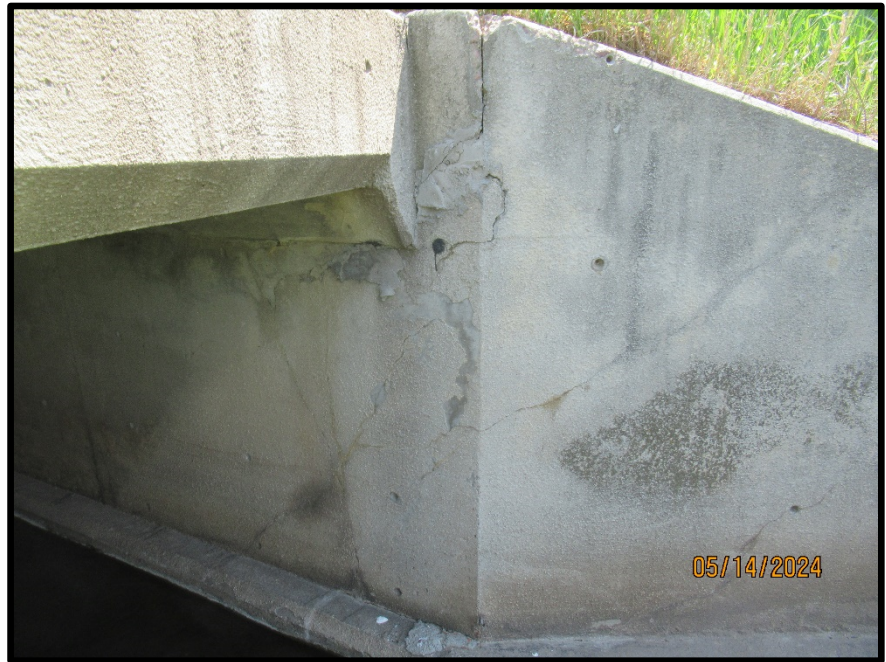
Cracking at SW Wingwall-Barrel Interface
