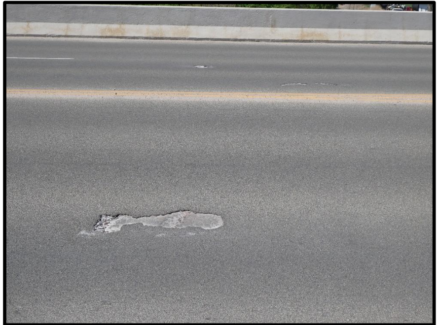
Spalls Through Chip Seal Overlay
