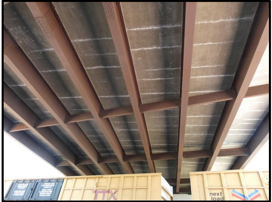
Typical Transverse Cracking with Efflorescence in Span 2
