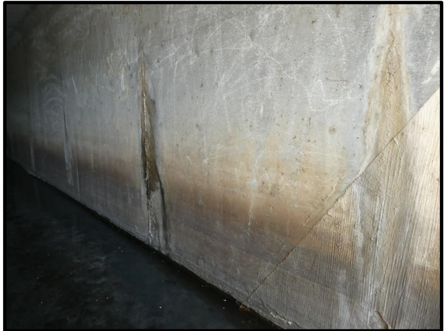
Vertical Cracking with Efflorescence and Leakage – North Wall of Barrel 3
