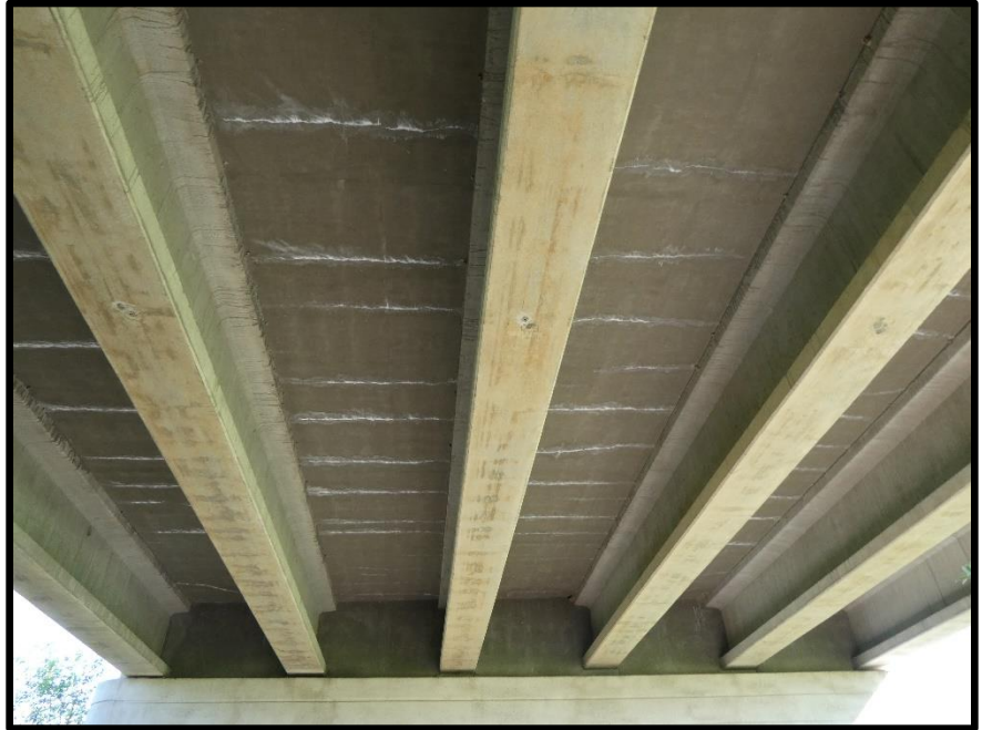
Typical Transverse Cracking to Underside of Deck – Span 1 Shown
