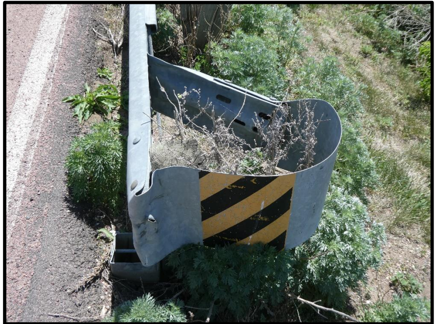
Collision Damage to NW Approach Rail End Terminal
