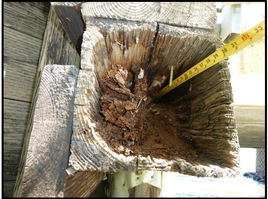
Decayed West End of North Abutment Cap
