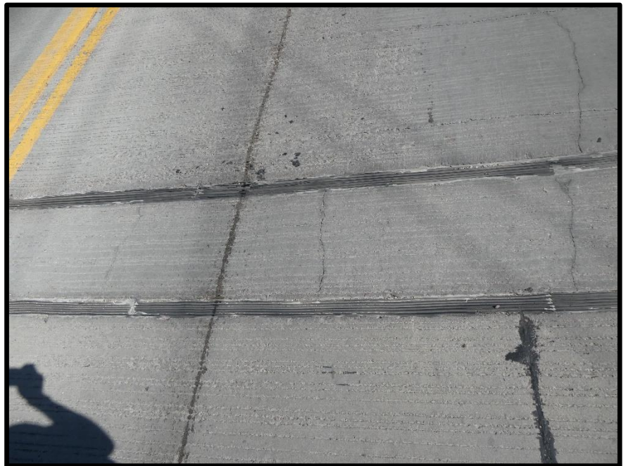
Minor Cracking in Sleeper Slab and Top Hat
