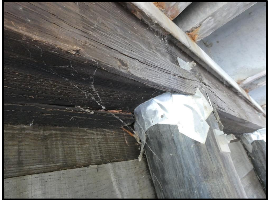
Crushing North Abutment Cap Over Pile 4 – Bottom View
