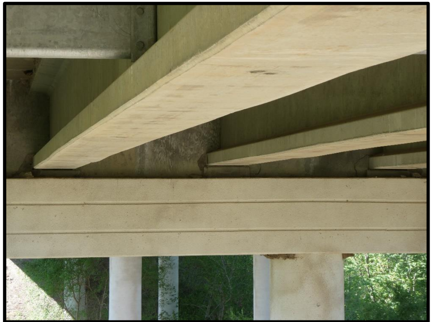
Typical Minor Spalls to Bent Diaphragms
