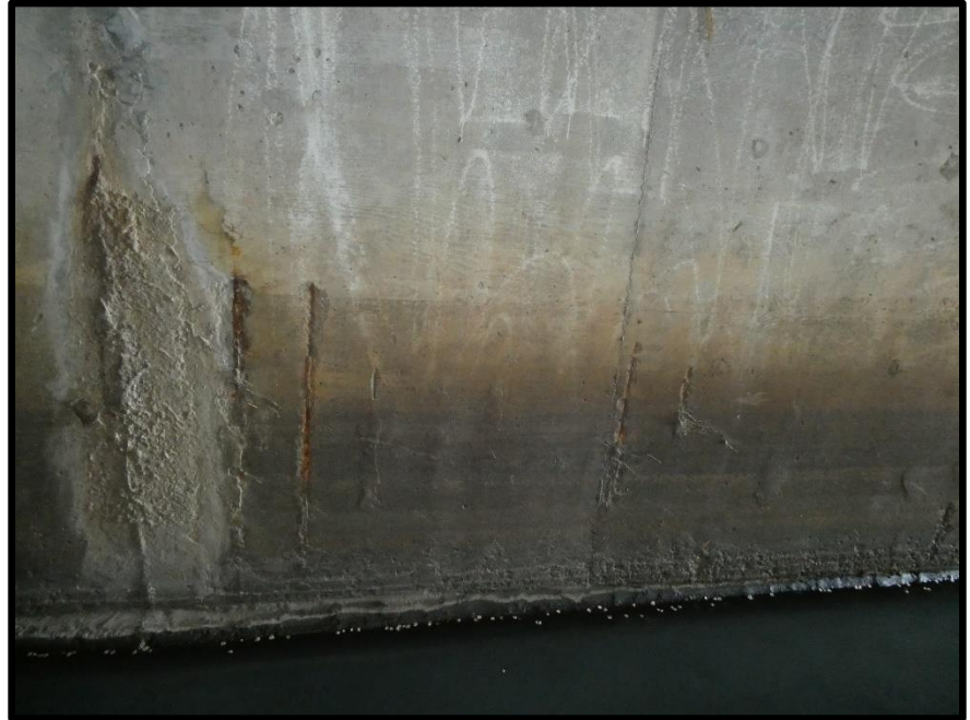
Exposed Rebar with Section Loss – North Wall of Barrel 3
